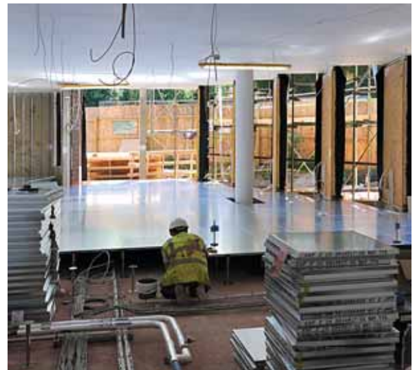
...the ground floor – all services run under the suspended floor...
